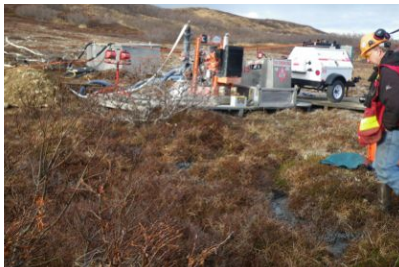
Figure 6. A visible trail of grey drill fluid was documented upwelling down gradient of the SUMP and flowing into a wetland. The last sump in a series of five is in front of the platform and pump.
